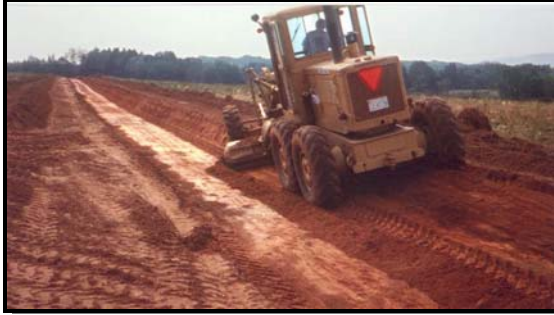
Soil excavated when forming the channel is used to construct the berm
